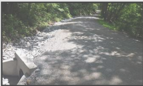
Hickory Nut Road: This Dirt and Gravel project replaced 7 cross pipes, added 4 new pipes, and installed new inlets and outlets. 1,386' of riprap lined ditches were added along with the re-establishment of 650' of roadside ditch. 365' of 18" HDPE storm pipe was used for the project.
