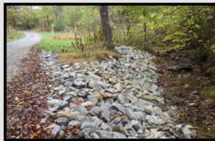
Ramage Road: This Dirt and Gravel project added 3 new cross drains with headwalls and R6 riprap energy dissipators at the outlet. Approx. 500' of roadway was raised 12-18". 75' of riprap streambank stabilization occurred adjacent to the roadway. 675' of riprap-lined ditches were added, using 90' of 15" HDPE storm pipe for the project.
